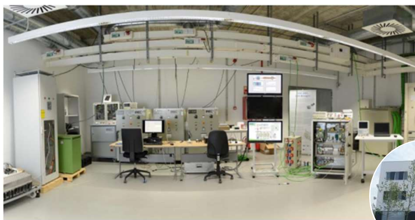
Base Barcelona: Smart Energy Lab
